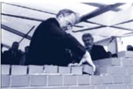
Uwe Wölfer, cosmed director, at the laying of the foundation stone for the new production facility of the Polish affiliate in Poznan, Poland
